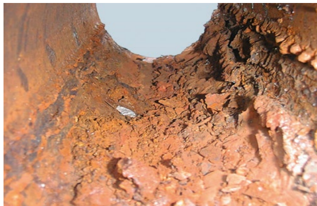
Corrosion on the inside of an untreated pipe
